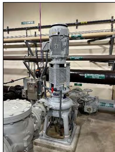
New Drain Pump No. 2
