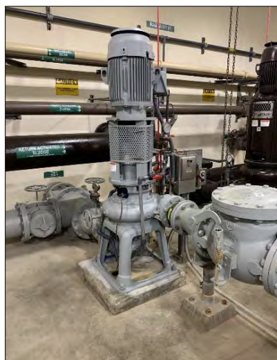
New Drain Pump No. 1
